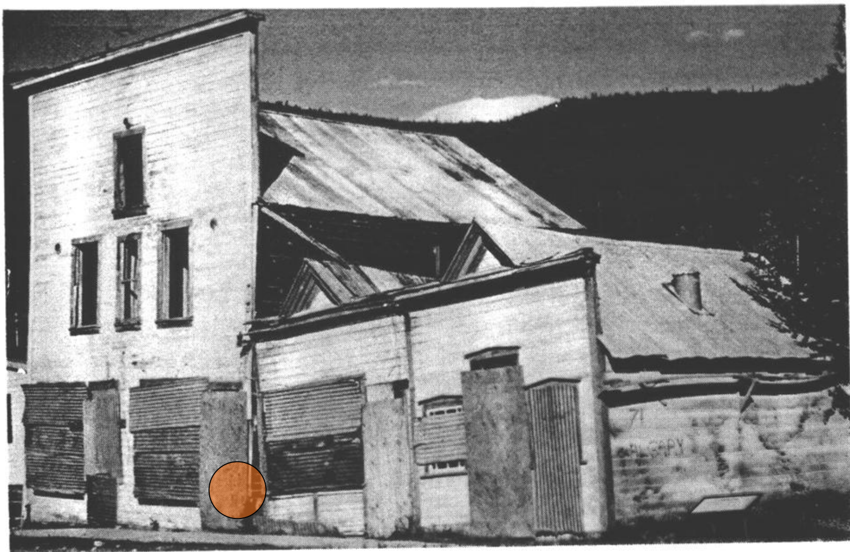
Plate II: Building Showing the Results of Thaw Settlement in Dawson City, Yukon Territory, Canada.
