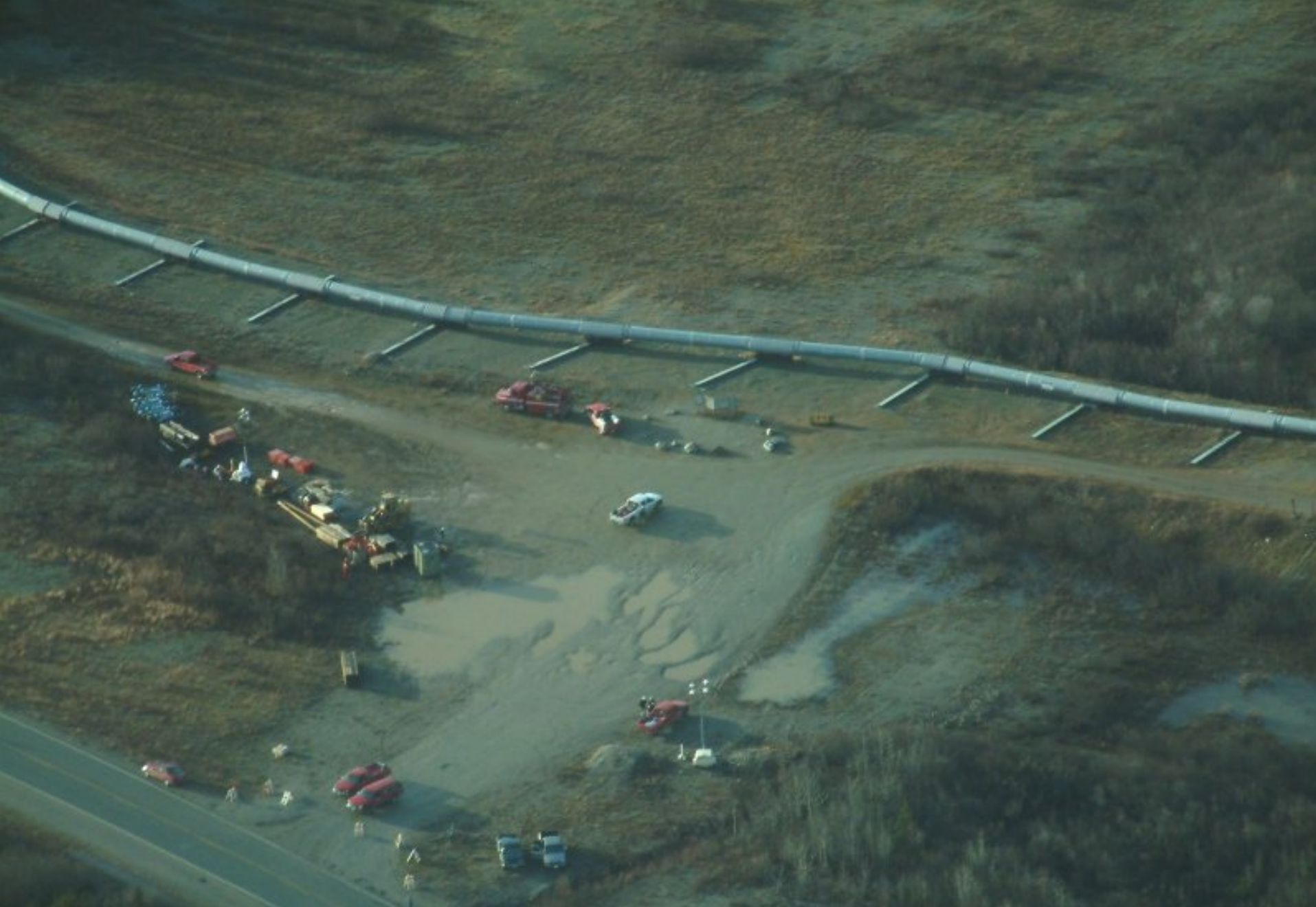
Trans-Alaska pipeline showing displacement and collapse
