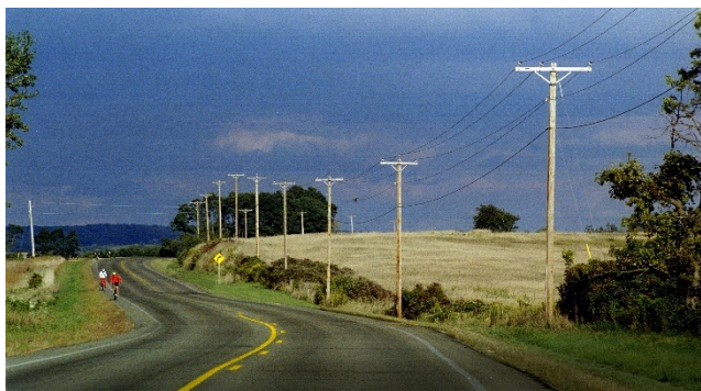
Medium voltage distribution lines
