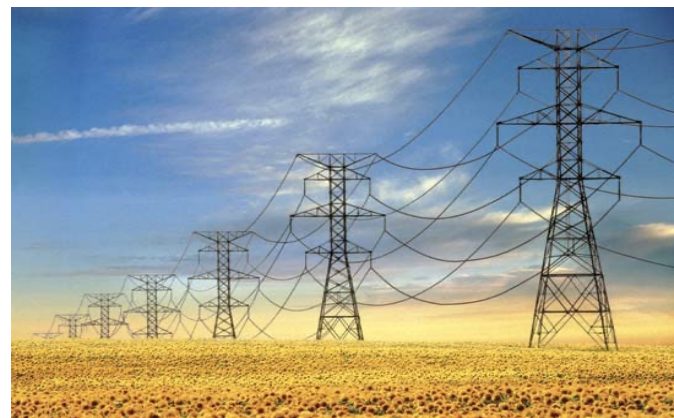
High-voltage power transmission
