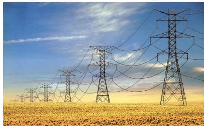
High-voltage power transmission
