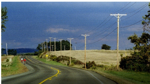
Medium voltage distribution lines
